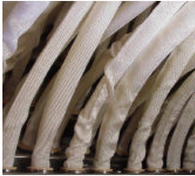
Drainage Loops Inside the Tank
